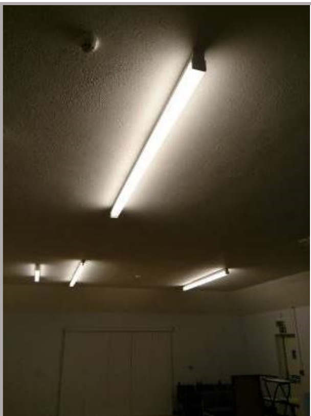
Figure 8 Fluorescent strip lights in the youth centre
