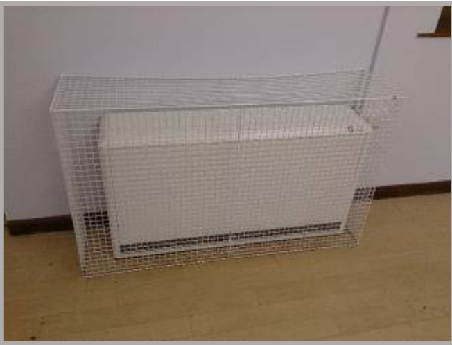
Figure 9 Electric storage heaters in the youth centre
