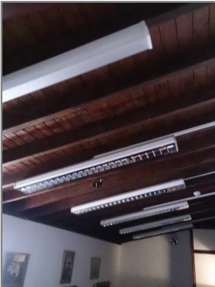
Figure 7 Meeting room lighting
