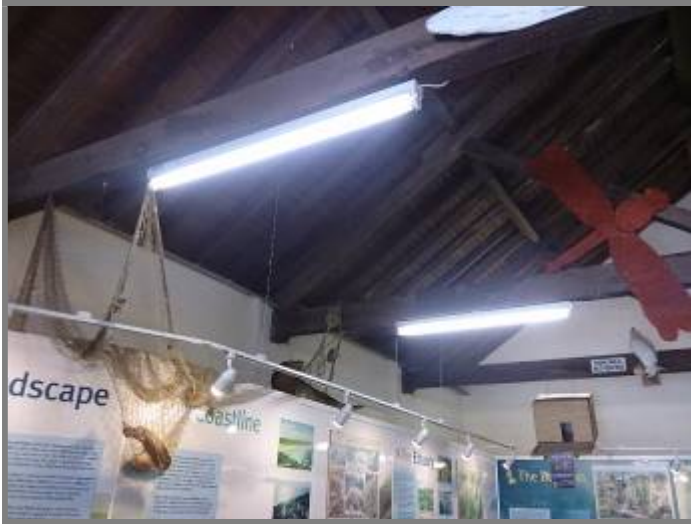
Figure 6 Main lighting and display lighting
