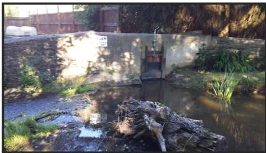
Figure 10 Top of the weir at low flow, with sluice gate at the top of the leat clearly visible
