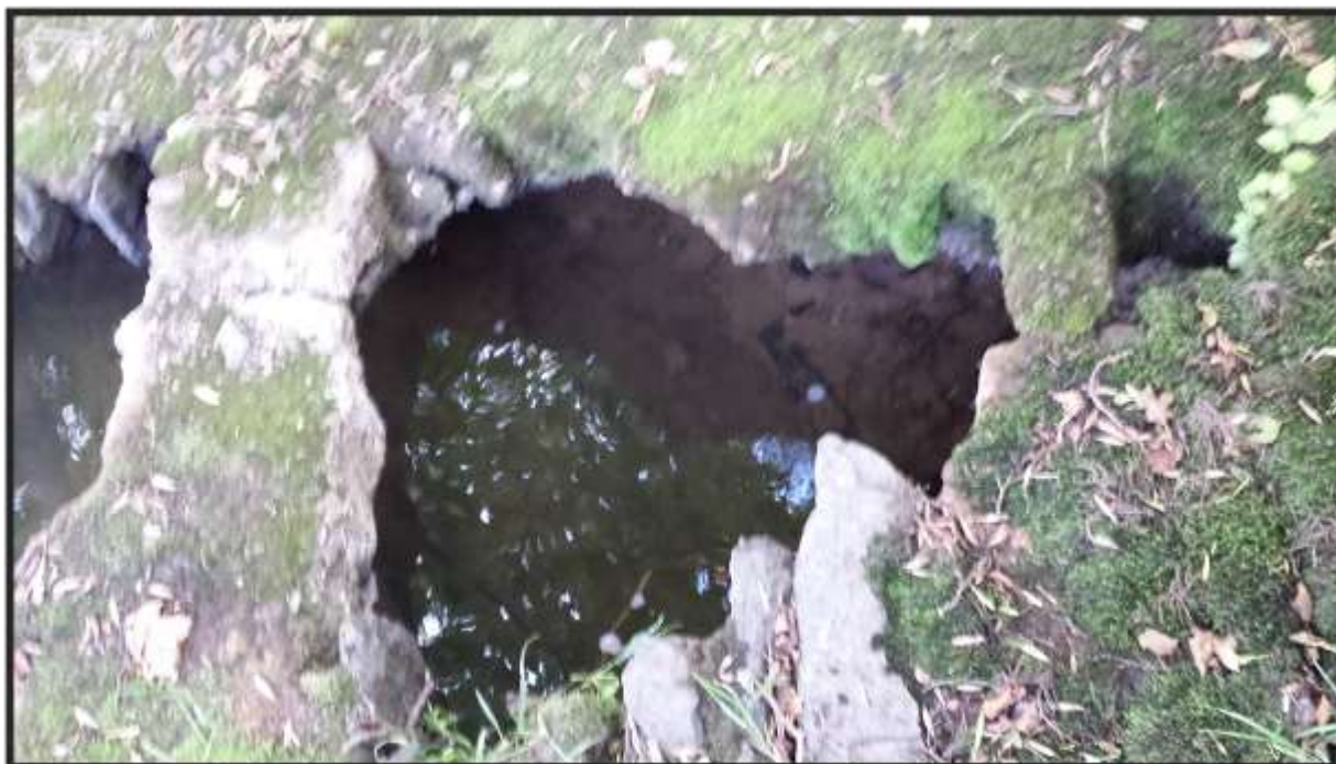
Figure 3 hole in the weir - poor condition
